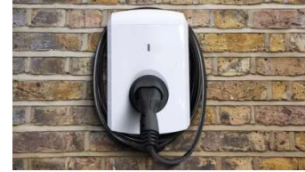
Figure 36: Electric Car charging
