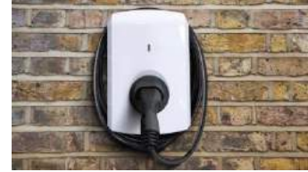
Figure 36: Electric Car charging
